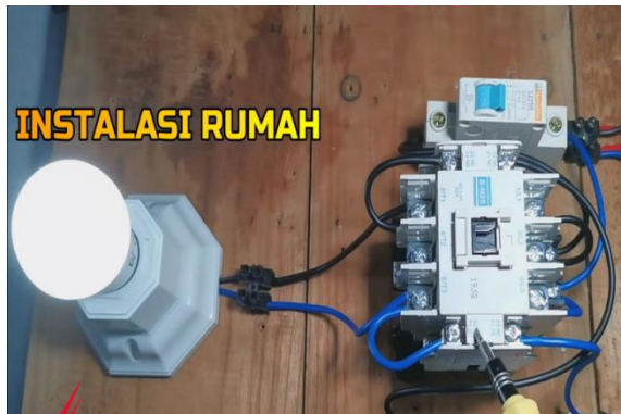
Gambar 4. Automatic Transfer Switch (ATS)
